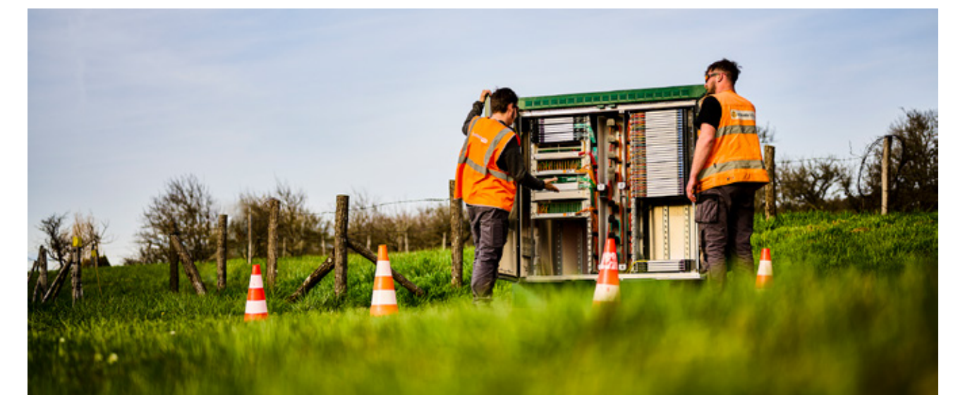
Spinnaker project, fibre optic network Infrastructure | Europe | Partner: Arjun
